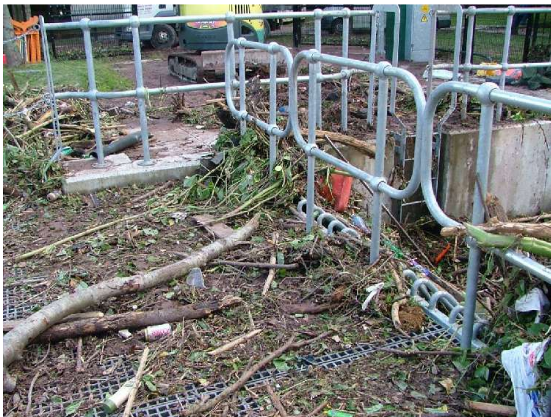
Church Street – Park – Trash Screen
