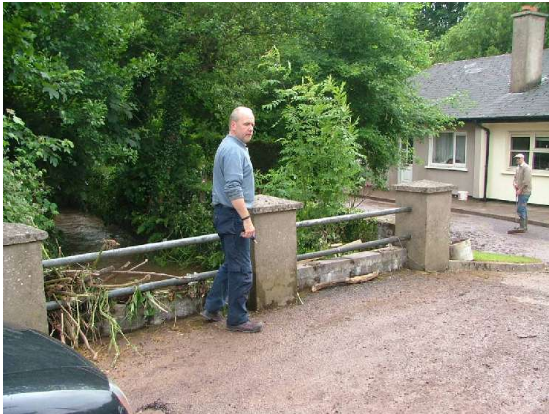
Residential Property – Behind Meeting Hall – Church Road – Bridge Blocked
